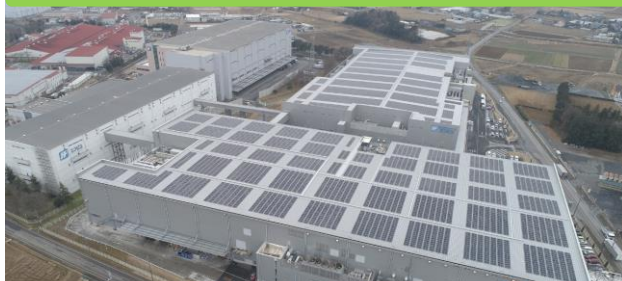
System for Kanto Recycling Plant Operation commenced in March 2022
